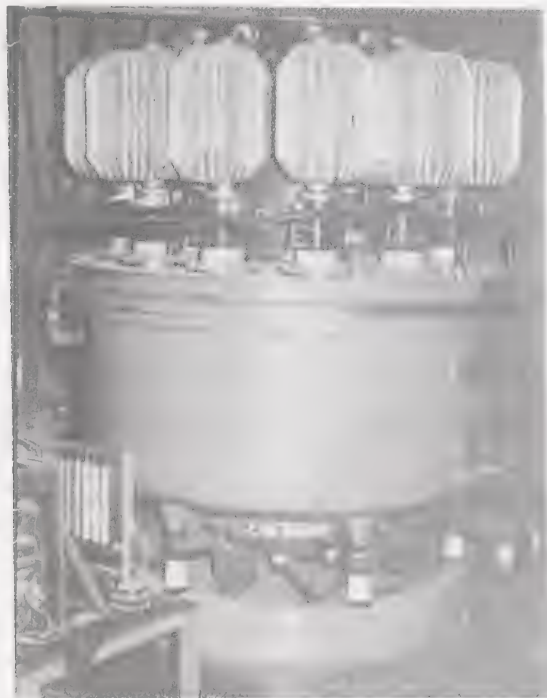
Plate 16. (Edmonton Power) 1929 Brown Boveri Mercury Arc Rectifier in 1981
